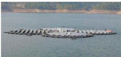
Fig. 1. Floating photovoltaic system in Korea, from [9].
