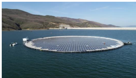
Fig. 1. The utilized FPV unit on the reservoir surface of the Banja hydro power plant.
